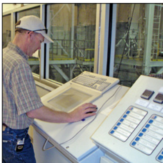
Custom PLC controls
